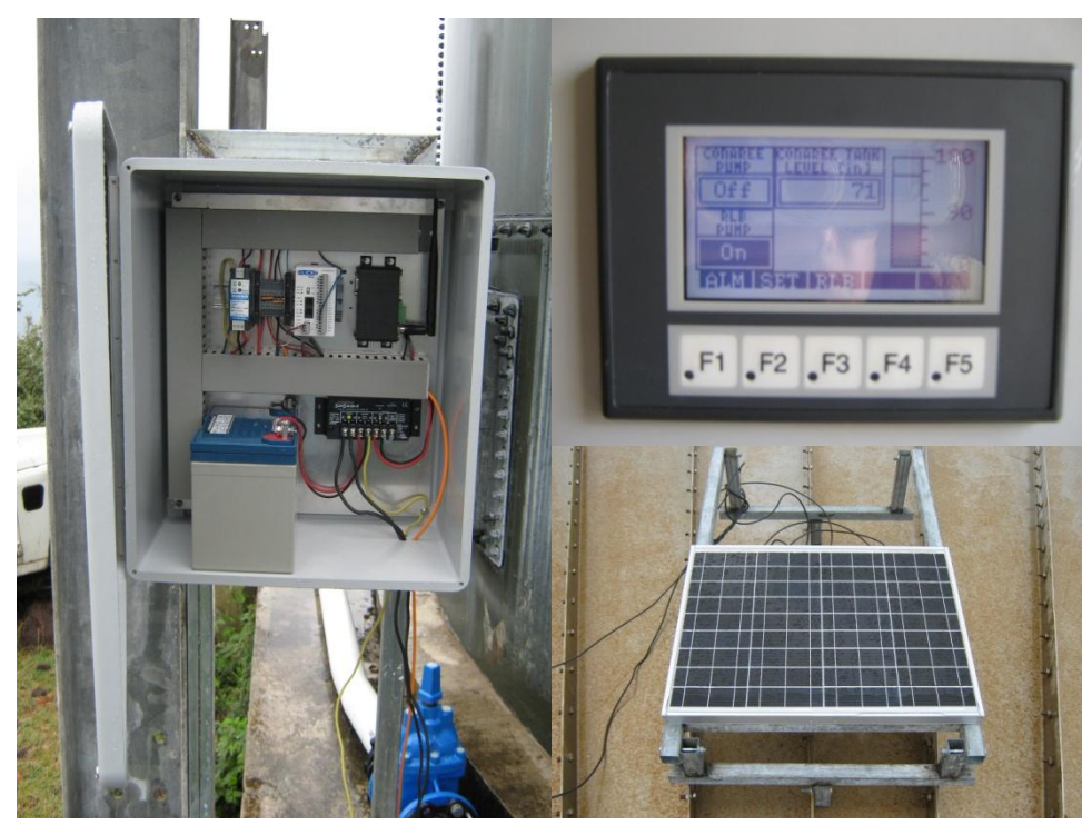
Installation of automated tank level controls to prevent overflowing of storage reservoirs
